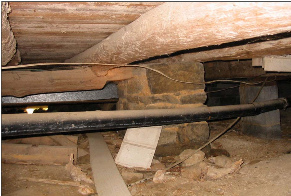
Figure 6. View of crawl space, showing stone pier and log joists and summer beam (History Matters, 2005).
